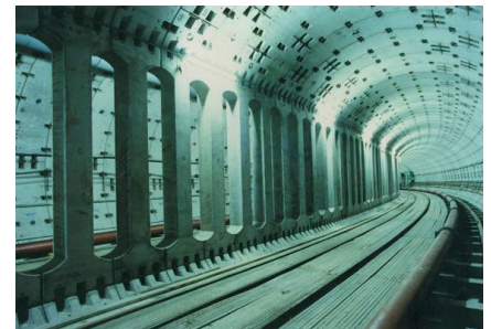
▲ Construction of a curved section of the Hiroshima Astram line (new transportation system) (radius: 135 m)
