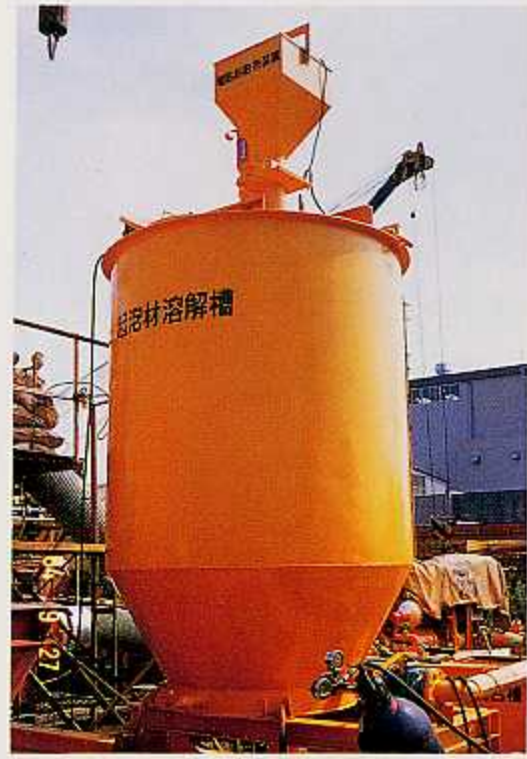
Foaming Solution Mixing Tank
