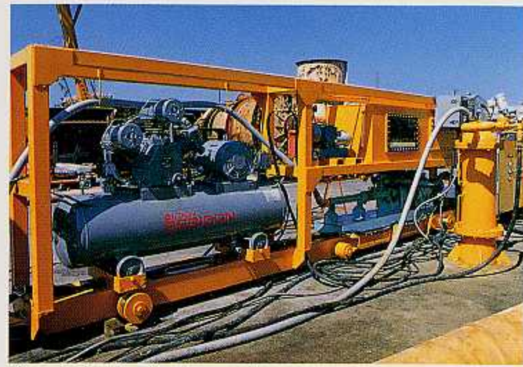
Foam Injection Equipment Car
